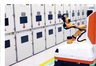
Robotic High-voltage Switchgear Operation
