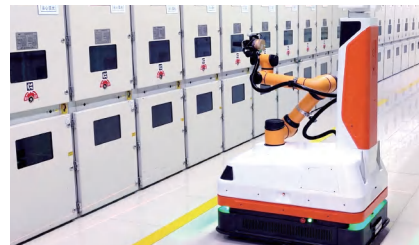
High-voltage distribution cabinet operation
